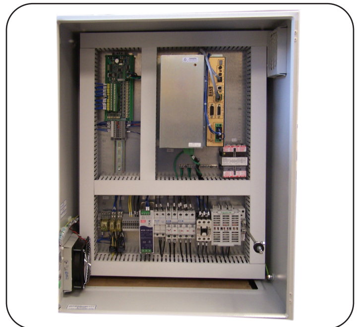
Inside View of the Enclosure
